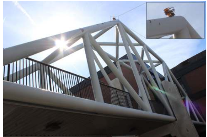
Fig. 19. The robot operates on a cylindrical steel bridge to perform thickness measurements and checking for corrosion.
