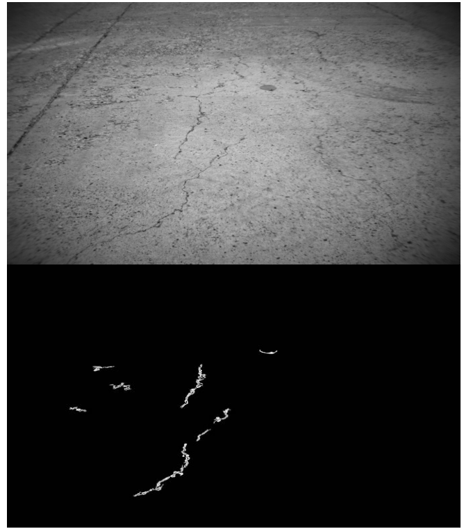
Fig. 3: An example image of the surveyed area (top), and an example output image from the crack detection algorithm with length filter applied (bottom).
