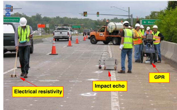
Fig. 1. The state-of-the-art of the NDE technology for bridge deck inspection and evaluation.
