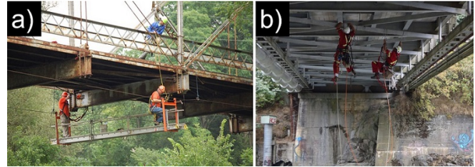
Fig. 1. Dangerous bridge inspection scenes, source: Harcon Corporation and Working AT Height Alti-Service™.
