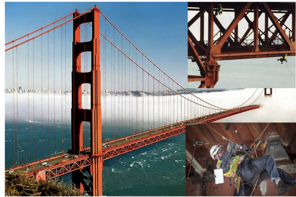
Fig. 1: Current practice of steel bridge inspection: rope certified bridge engineers inspecting the Golden Gate bridge, San Francisco, California [3], source: NBC April 2018.
